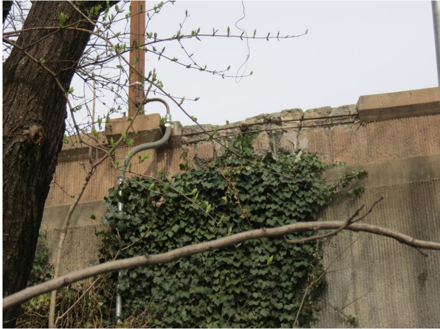
IMPACT DAMAGE APPR. "A" END RT. SIDE EBL
