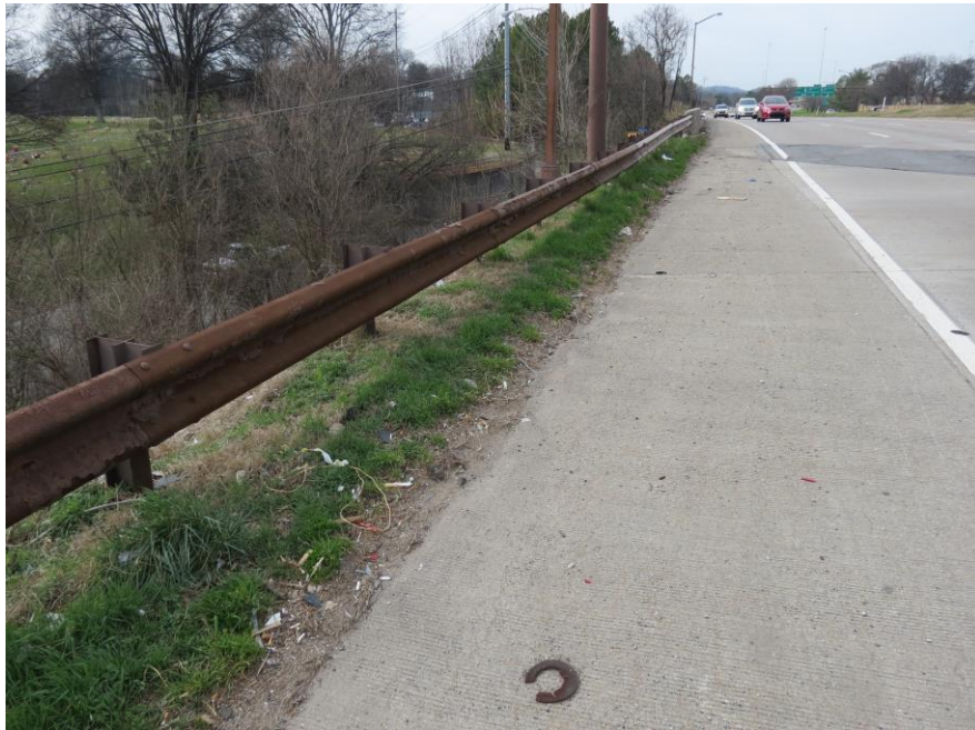
GUARDRAIL AT APPR. "B" END RT. W/ RUST EBL
