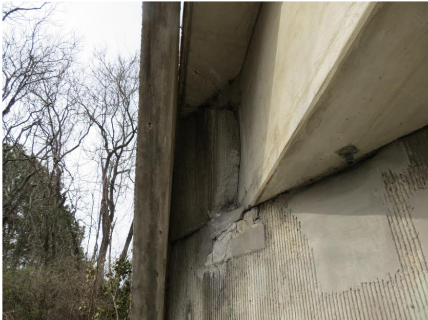
RT. WING ABUT. #1 W/ TILT & MISALIGNED
