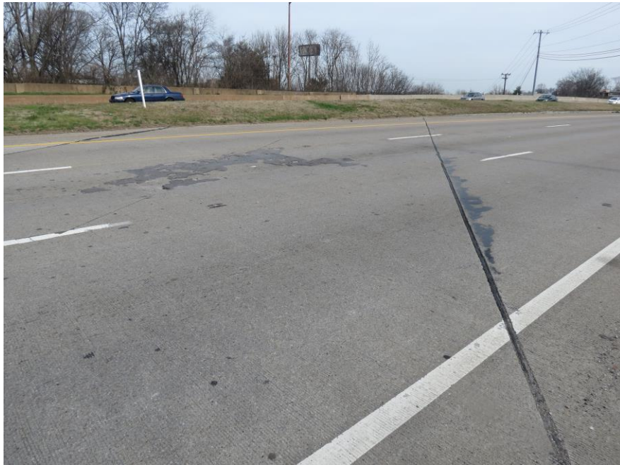
APPR. "A" END ROADWAY W/ PATCHES EBL
