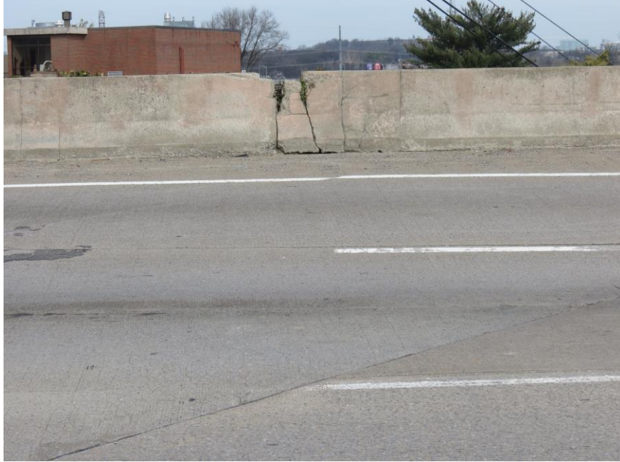
BRIDGE PARAPET "B" LT . W/ IMPACT DAMAGE WBL
