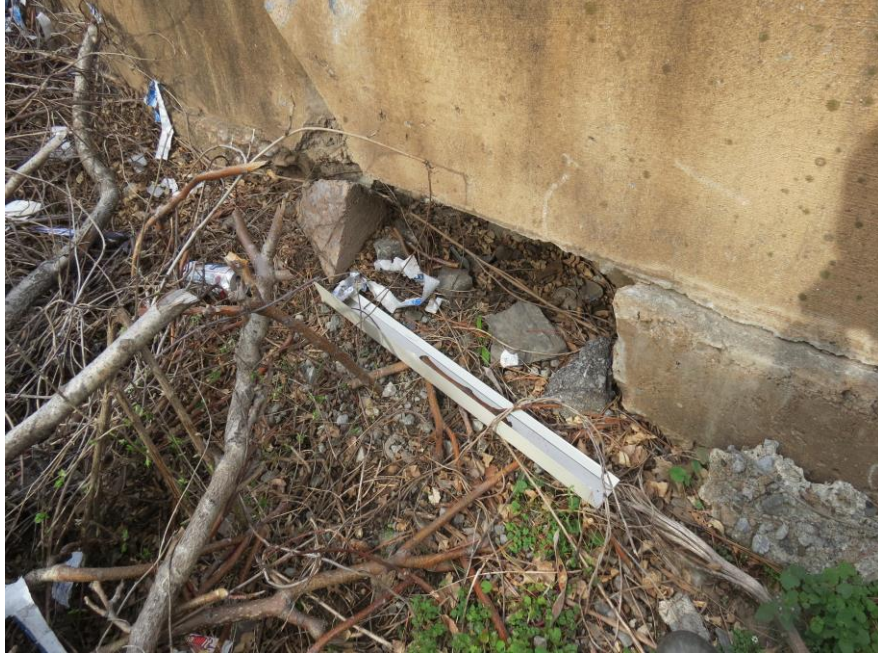
APPR. "A" END RT. SIDE W/ EROSION EBL
