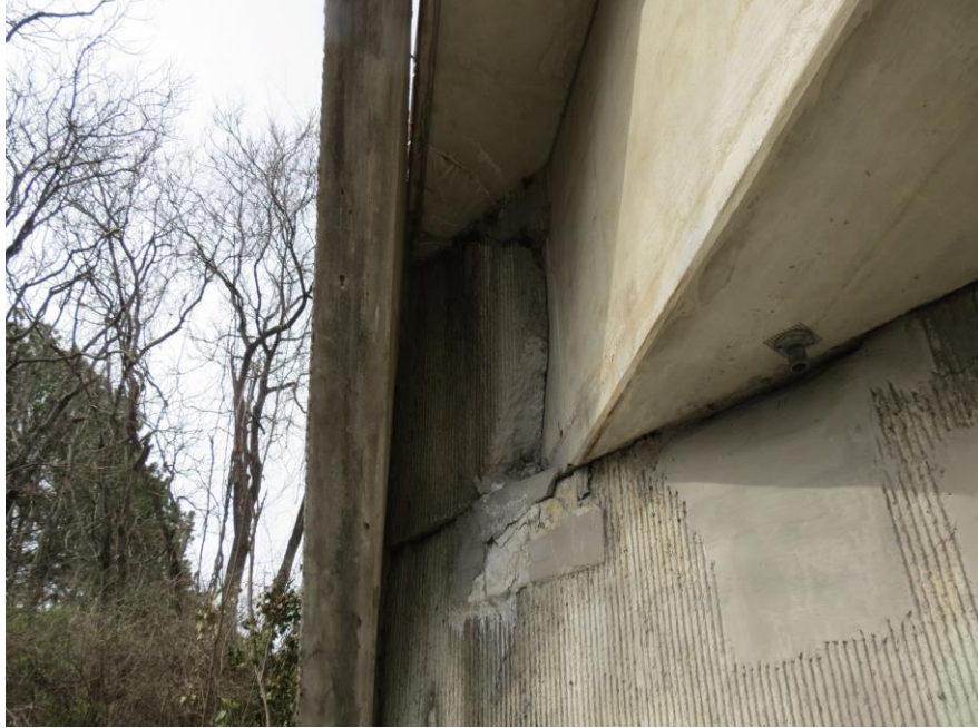
ABUTMENT #1 WALL W/ PATCHES AND SPALLS
