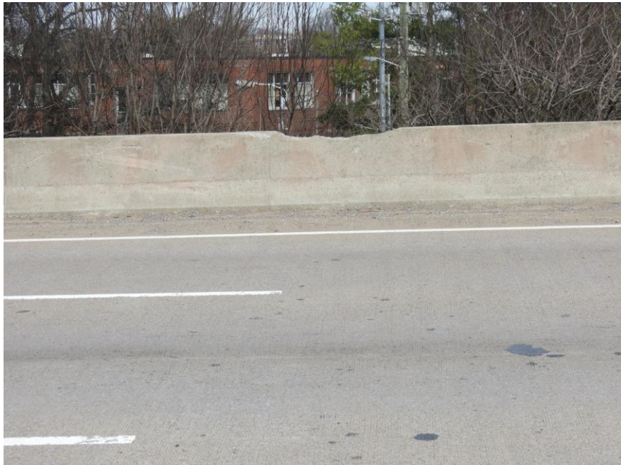
BRIDGE PARAPET LT. SIDE W/ IMPACT DAMAGE WBL
