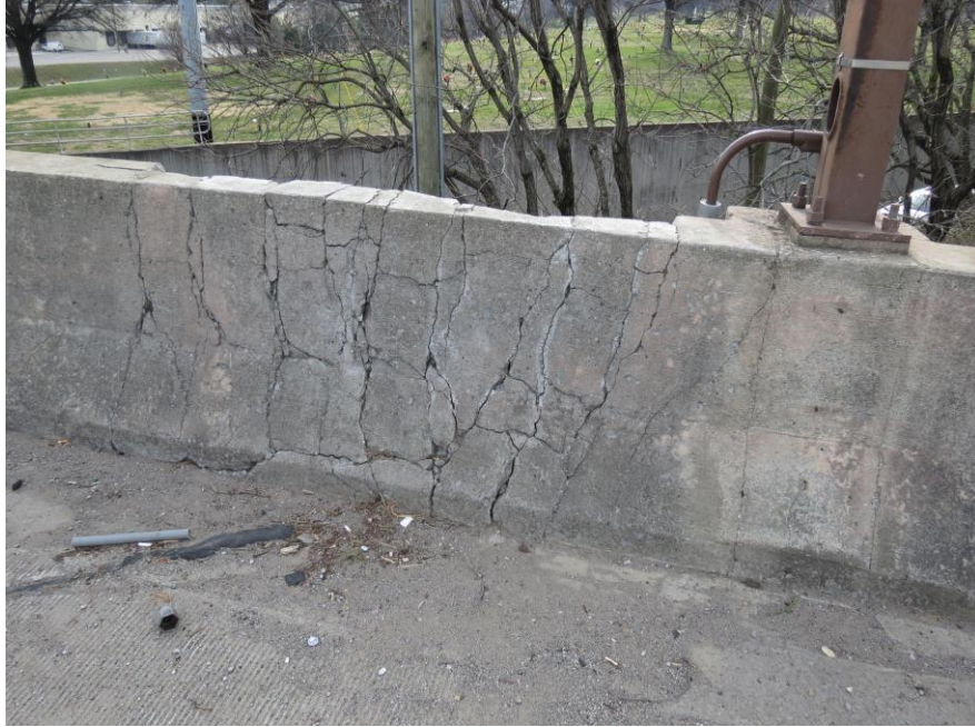
BRIDGE PARAPET "A" RT. W/ IMPACT DAMAGE EBL
