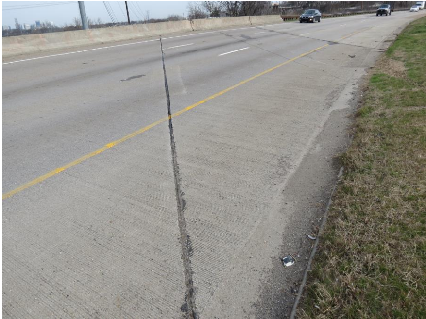
APPR. "B" END JOINT W/ TORN FILLER WBL
