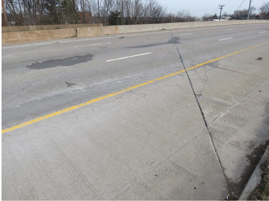
APPR. "A" END ROADWAY W/ PATCHES WBL
