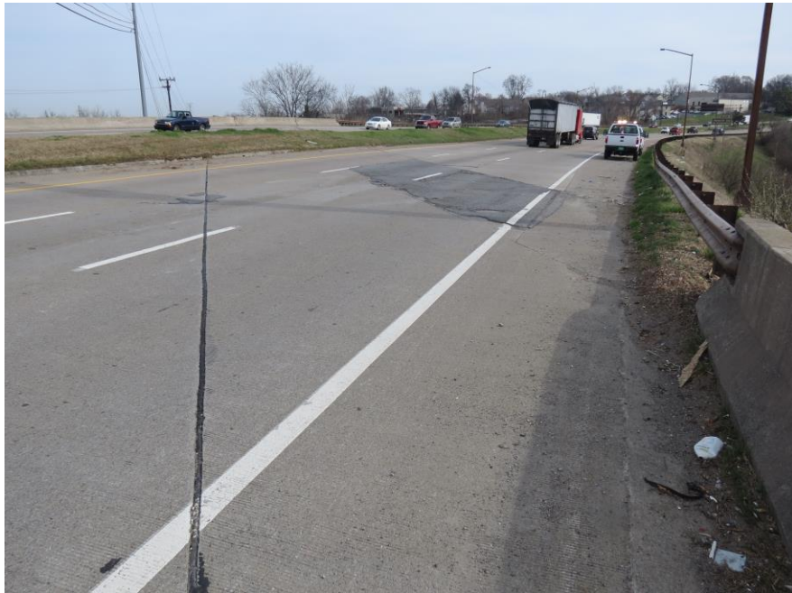
APPR. "B" END JOINT W/ TORN FILLER EBL
