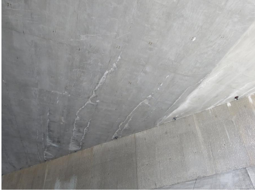
UNDERSIDE AT ABUT. #2 W/ OPEN CRACKS & EFF.
